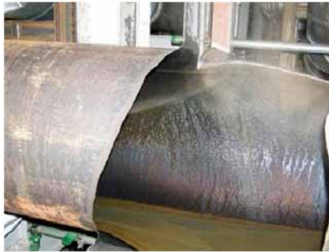
Figure 3. Steam line rupture caused four deaths
