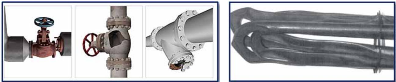
Figure 1-1. Piping and heat exchanger tube damage caused by water hammer
