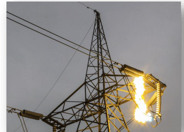
Catastrophic failure due to insulator defects
