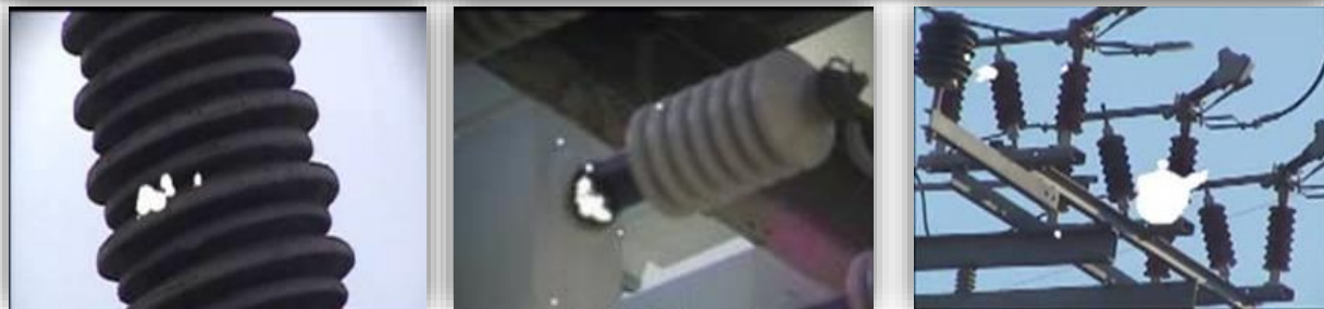
Early detection of faults in power systems using Ofil's camera
