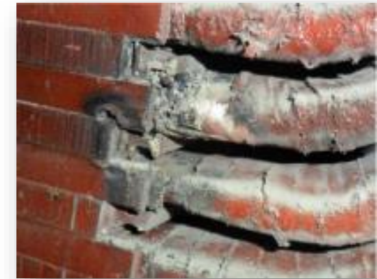
Motor Insulation failure due to PD
